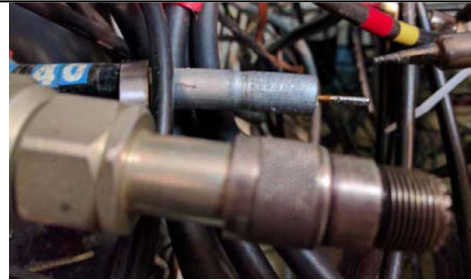
Photo 2: The hardline on the bottom (nearest the camera) is 1/2-inch 75 ohm, ends with a stinger into an N-connector, and then is adapted to a UHF-connector. The hardline on top is 1/2-inch 75 ohm. Previously it ended with a stinger into a commercial UHF-connector, but, as noted, two of the four the fingers of the UHF adapter broke. Also shown is a soldering iron tip, depositing solder on the center conductor ("tinning" the center conductor). This will make it easier to "fatten" the center conductor by using a salvaged part from a PL-259. See photo 3.
